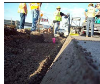
b Angular Cold Joint.
