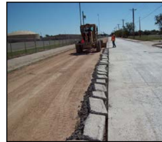
a Vertical Cold Joint.
